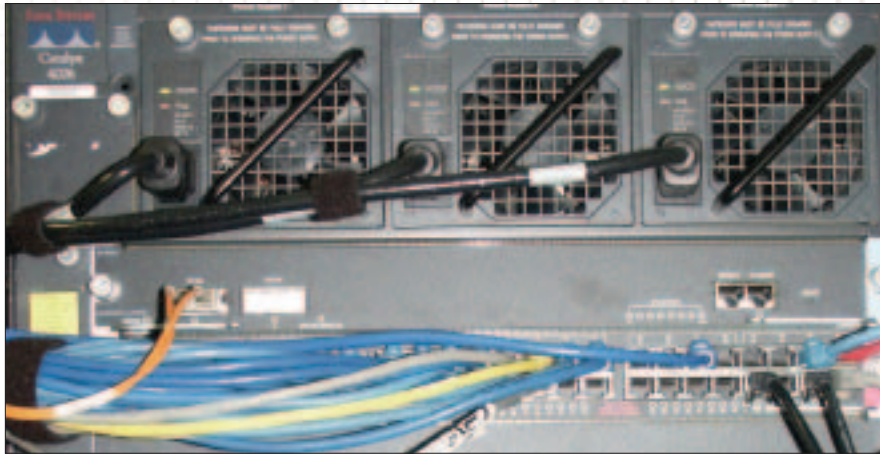
Redundant, hot-swappable devices in critical hardware keeps the network humming while awaiting repairs.
