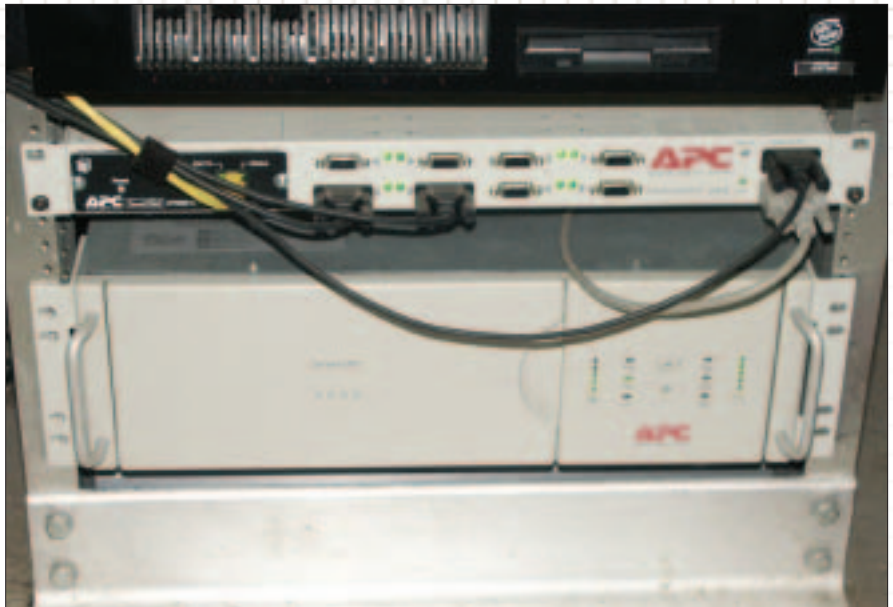
Servers should be connected to an uninterruptible power supply. During a power outage, the battery backup allows the server to shut down normally to prevent data loss.
